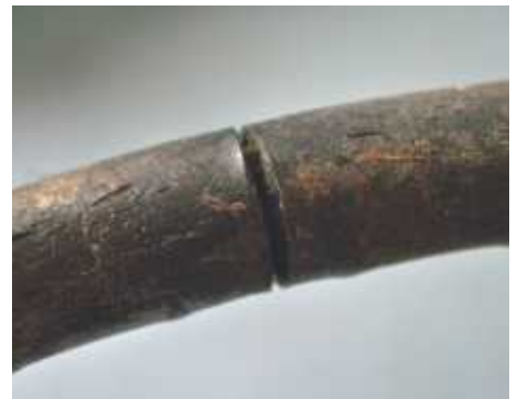
3 This crack goes all the way around the steel core and will need cleaning back to good metal.
