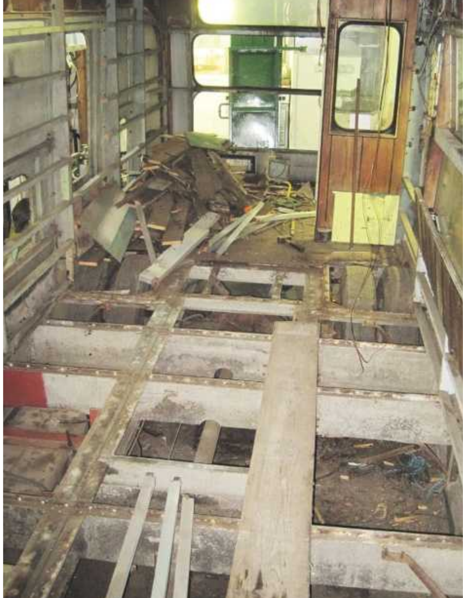
▲ The Beadle’s interior, stripped bare and exposing the alloy underframe before Ray Walsh began rebuilding work.
